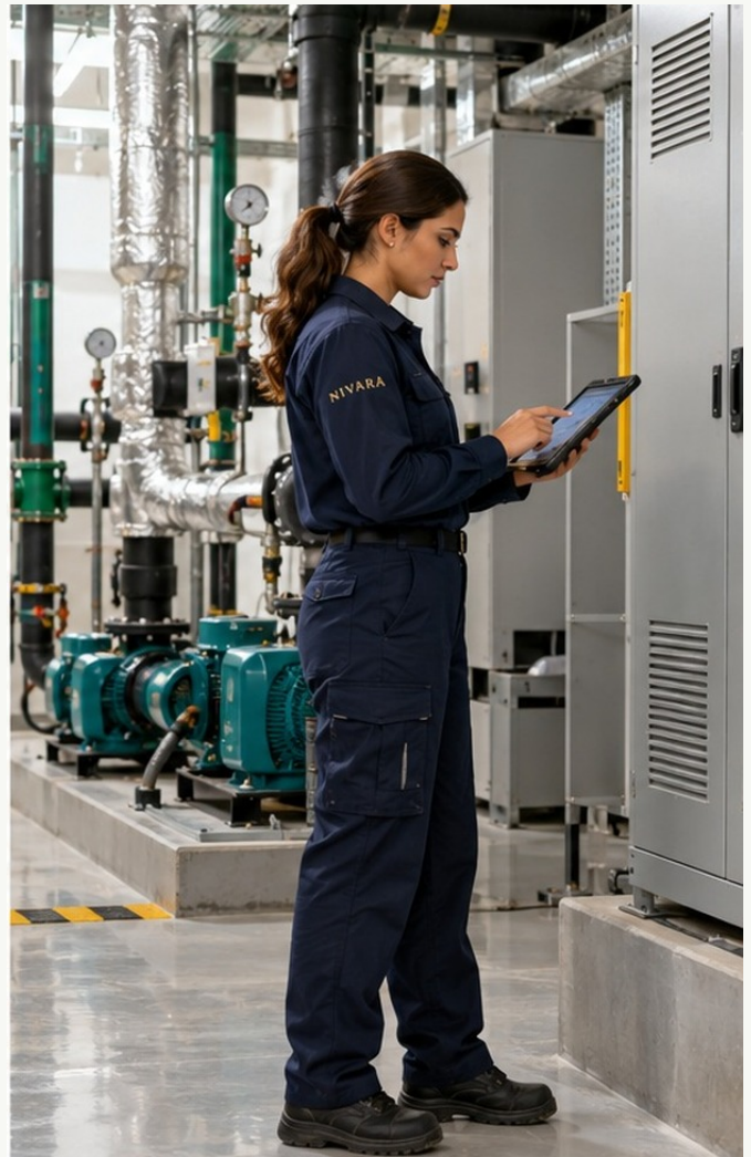
Equipment inspection and follow-up
