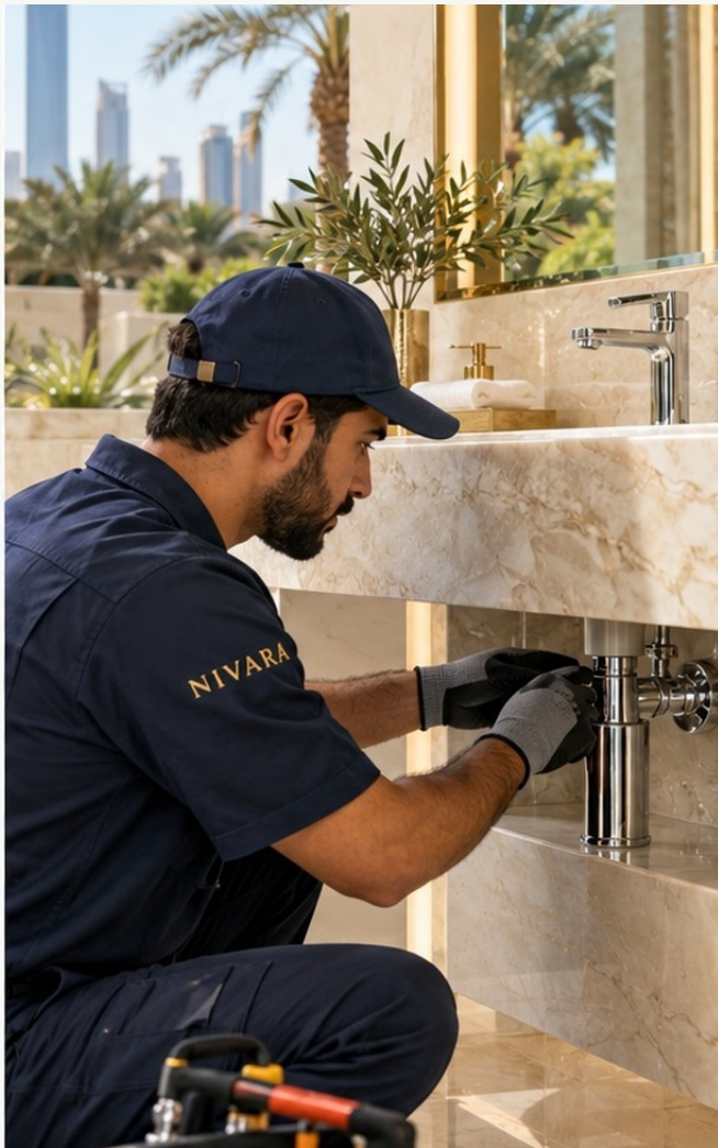
Plumbing and service coordination
